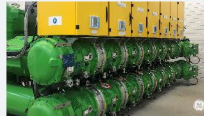
SF6-free switchgear in Norway
